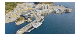
Northern Lights CO 2 receiving terminal (Under construction in Øygarden, Norway) (Image provided by Northern Lights JV DA)
