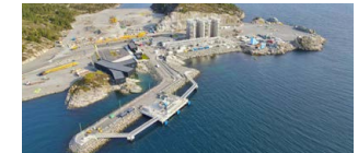
Northern Lights CO 2 receiving terminal (Under construction in Øygarden, Norway) (Image provided by Northern Lights JV DA)
