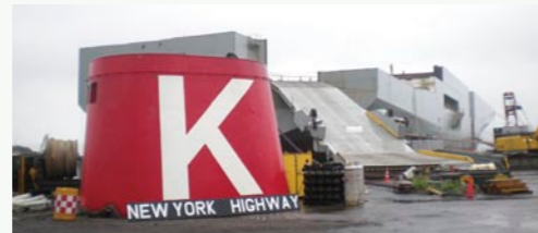
The funnel of the New York Highway that was removed (front) and the ship being demolished (back)
