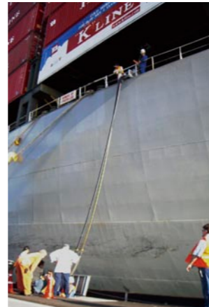
Power supply cables dropped from the ship (to be connected to the connection box)
