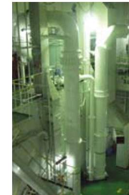
Pipelines for ballast water treatment system
