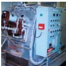
Waste Oil incinerator
