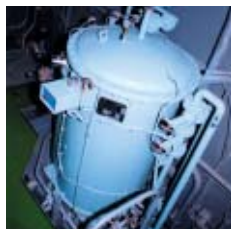
Oily water Separator
