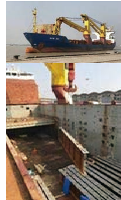
Unloading bridge girders from a break bulk vessel with a crane on our ship.
