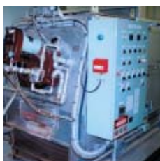
Waste Oil incinerator
